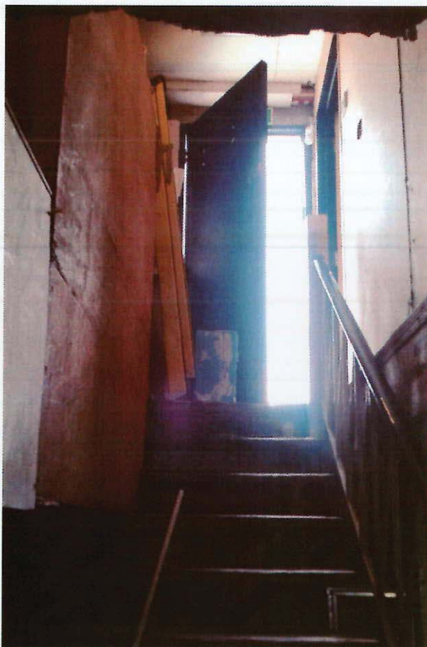
15. Basement – Looking up the stairs leading from the basement towards fire exit.
